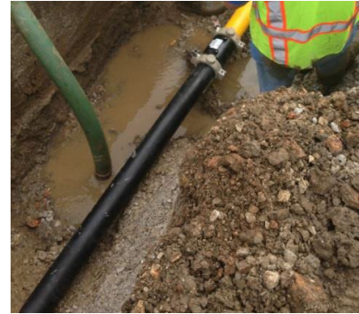
Figure I-a – Portable submersible pump (not visible)
